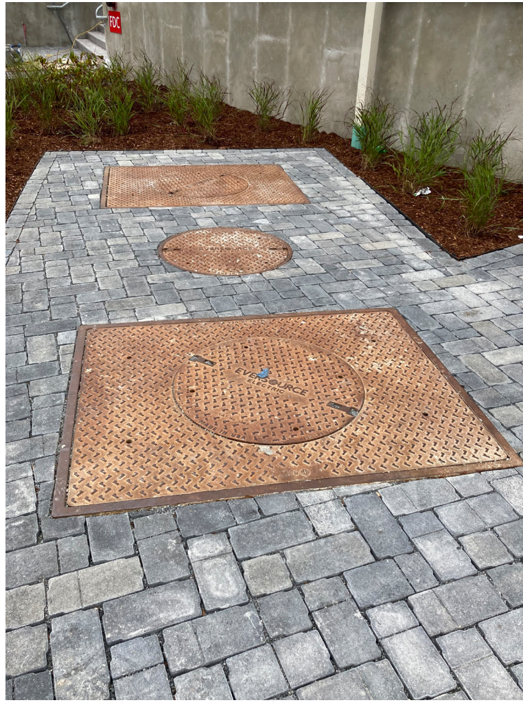
Permeable Pavers Around Utility Vault
